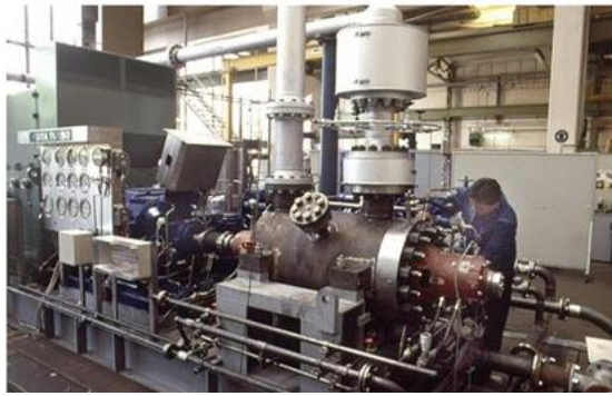
Gambar 4. Boiler feed pump
